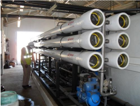
DESALINATION PLANT PIPING CELLS – SEP 2011
