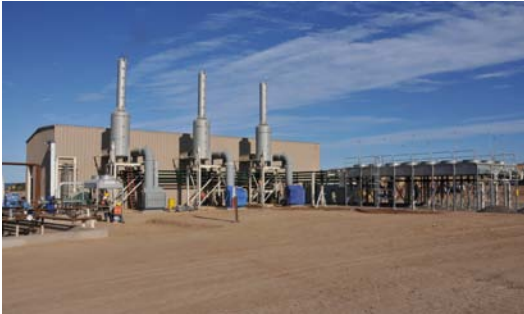
POWER GENERATOR– DEC 2011
